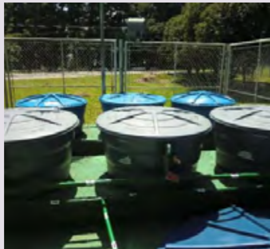
Curitiba: Waste water treatment plant
