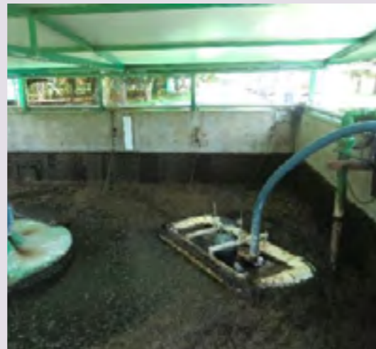
Station for treatment of effluents
